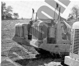
GRADERS at new school site prepare ground for excavation later this month.
